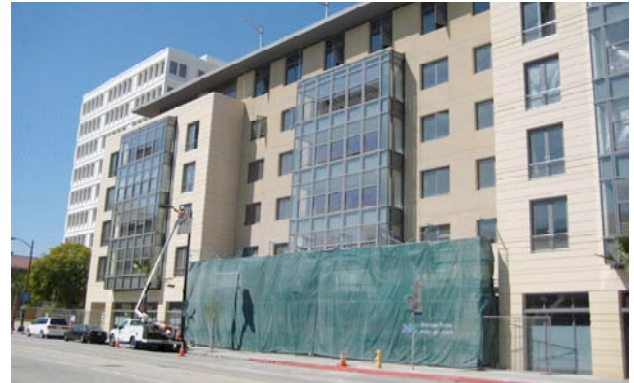
Photograph of the front façade of The Montana with covering over the area where Murrill is working on the façade. March 2008.
